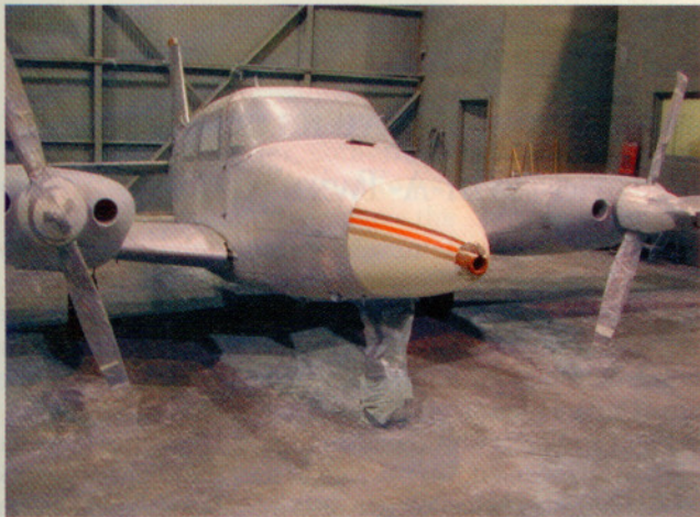
The first pass blew all the old paint off the airplane's aluminum skins. The fiberglass nose cone will get its own paint-removal treatment. Looks better already!
